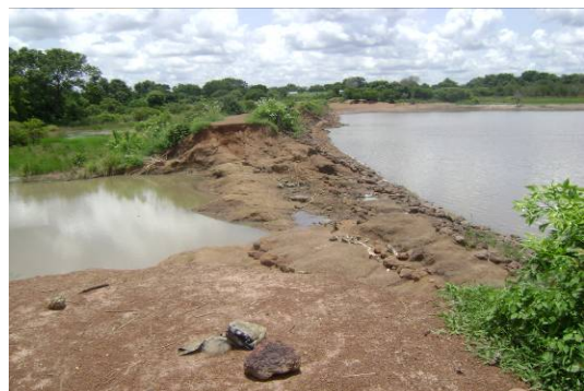
Plate 4: Broken Dam at Piina
